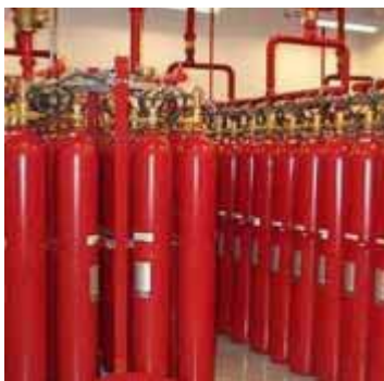
Fire suppression system
